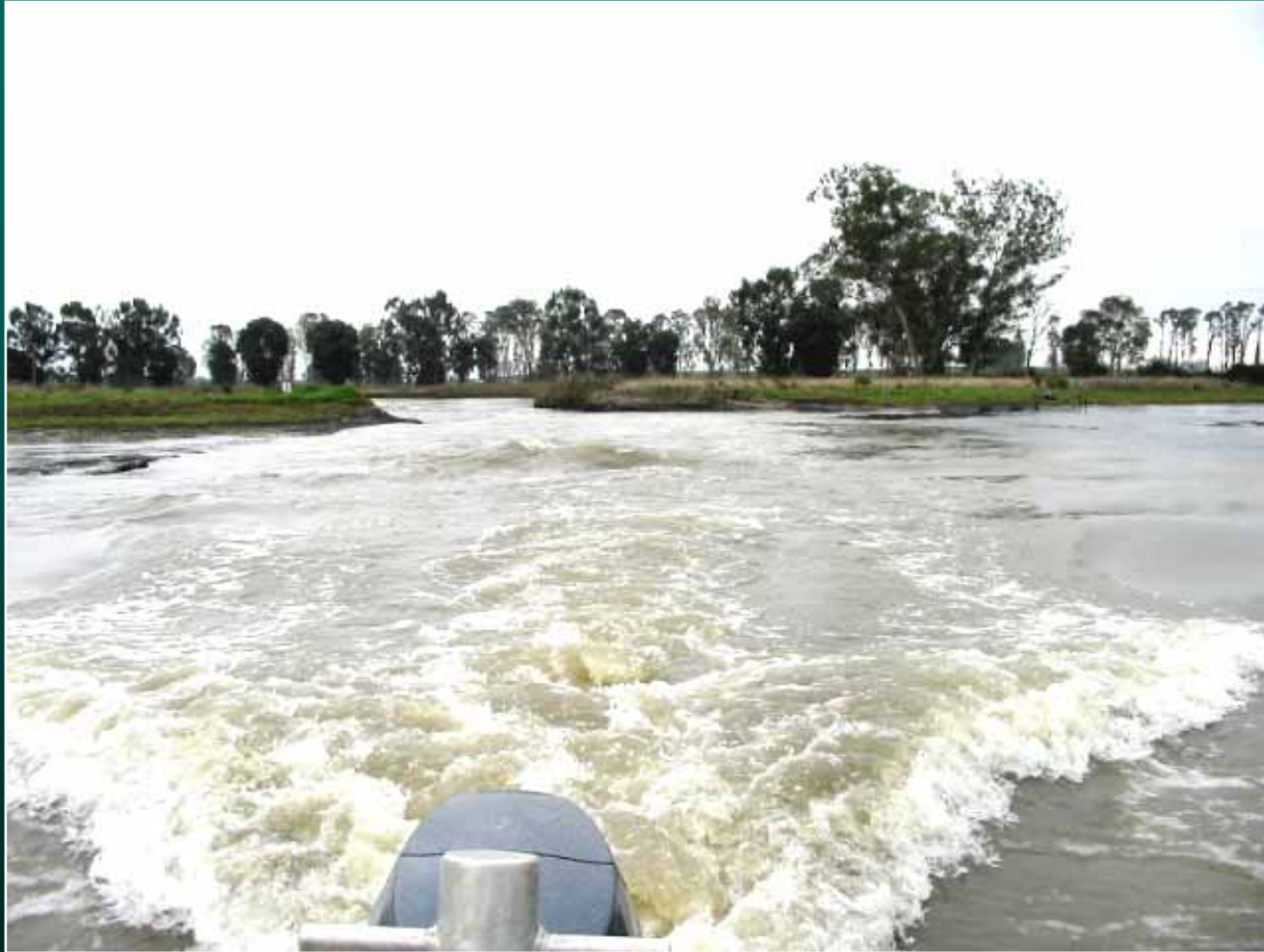
SWOA levee breach, March 2004.
